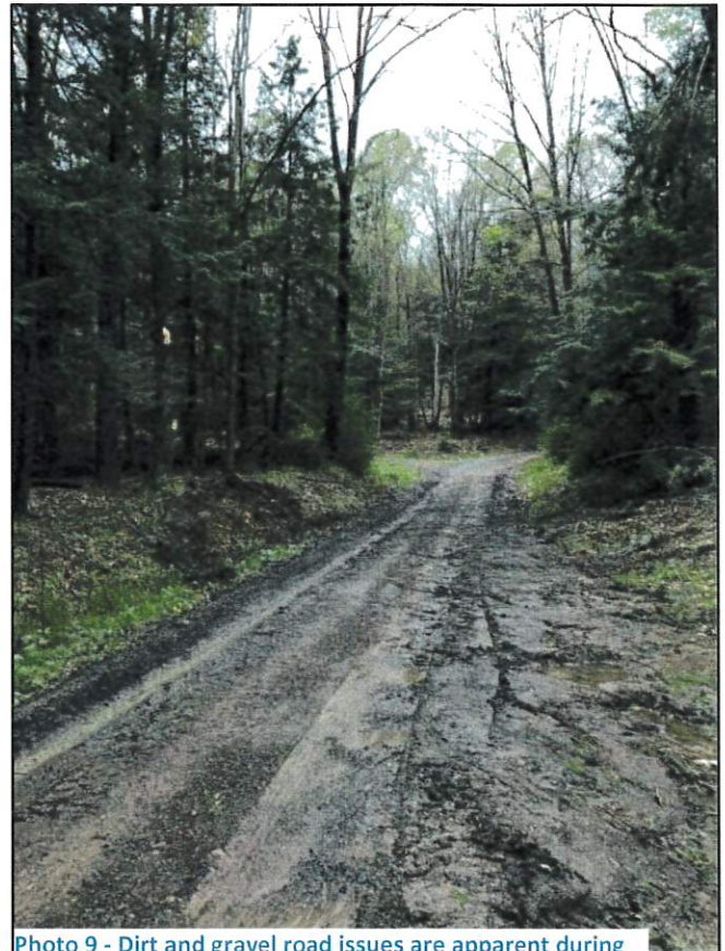
Photo 9 - Dirt and gravel road issues are apparent during or immediately following heavy rain events
