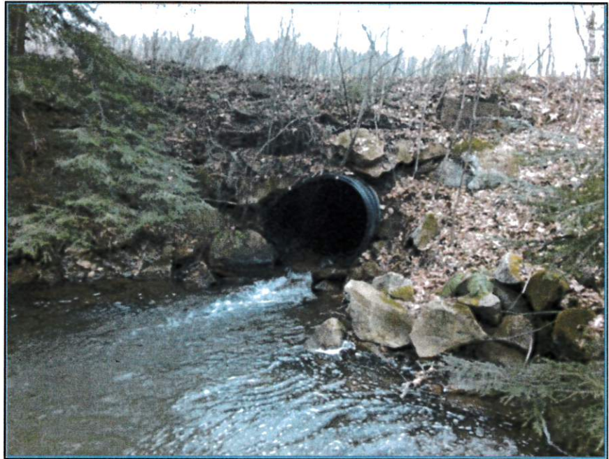
Photo 13 - An undersized culvert on Keal Run in need of replacement
