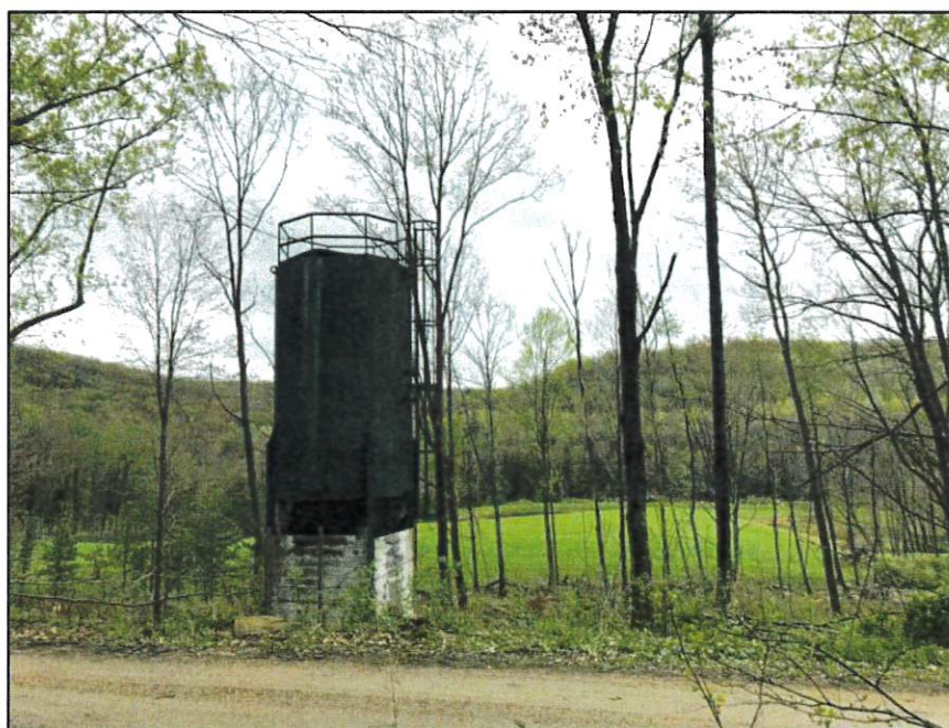
Photo 5 - A limestone dosing silo treating an AMD discharge on the South Branch
